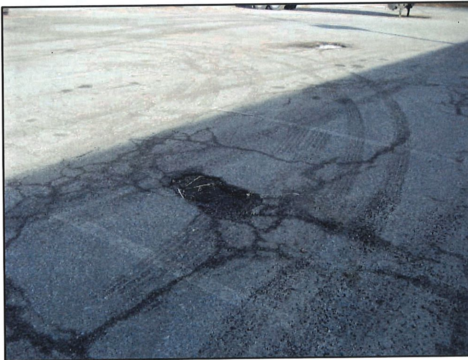
Photo 2 – Engineering Control C-2: Asphalt Cap Protective of Human Health and the Environment, but in need of repair
