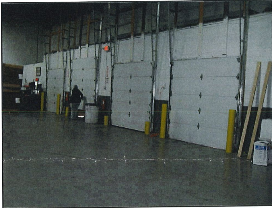
Photo 9 – Engineering Control C-3: Concrete Slab (Building Foundation) Protective of Human Health and the Environment
