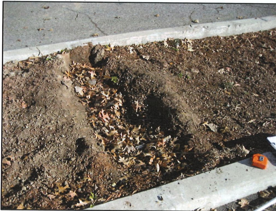
Photo 11 – Engineering Control C-4: Vegetative Cap Protective of Human Health and the Environment but in need of repair
