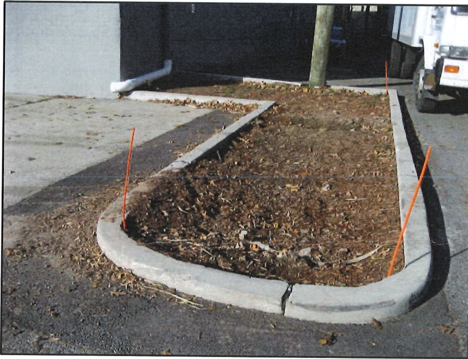
Photo 11 – Engineering Control C-4: Vegetative Cap Protective of Human Health and the Environment but in need of repair
