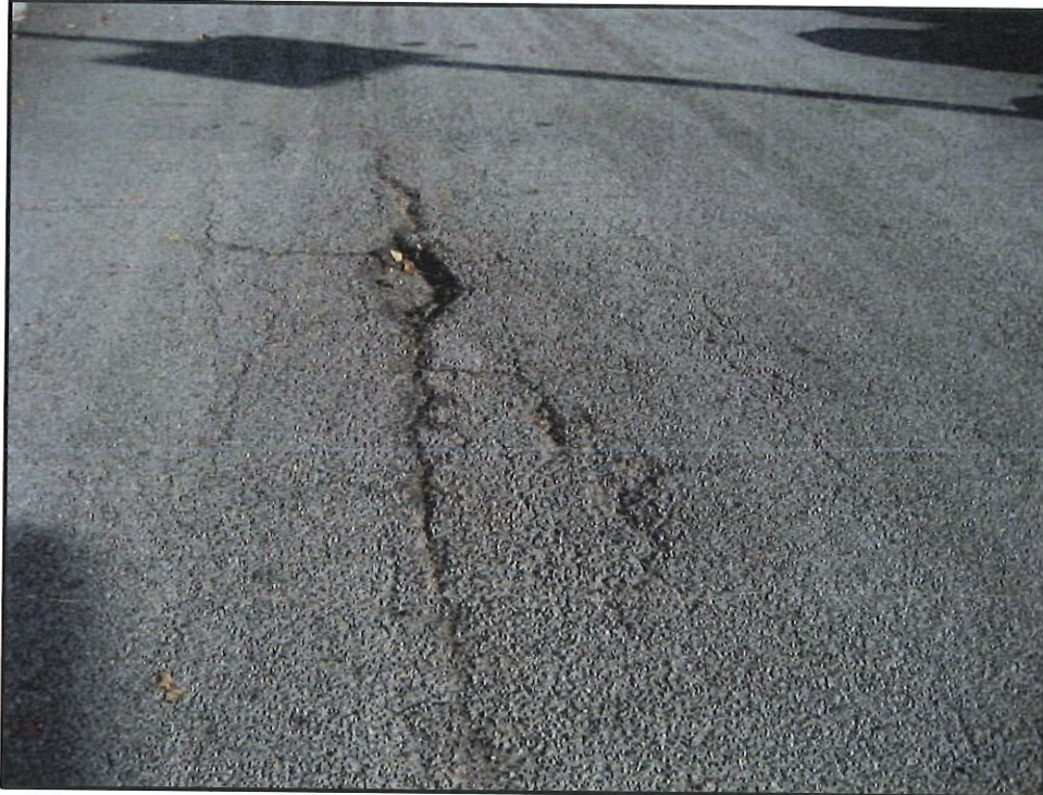
Photo 3 – Engineering Control C-2: Asphalt Cap Protective of Human Health and the Environment, but in need of repair
