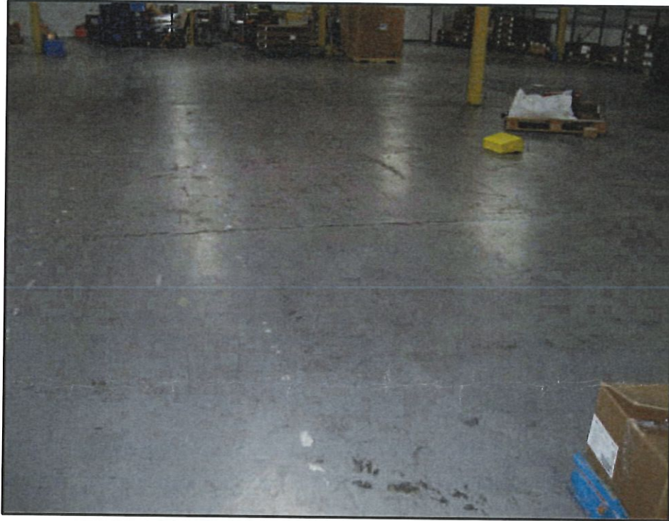
Photo 7 – Engineering Control C-3: Concrete Slab (Building Foundation) Protective of Human Health and the Environment
