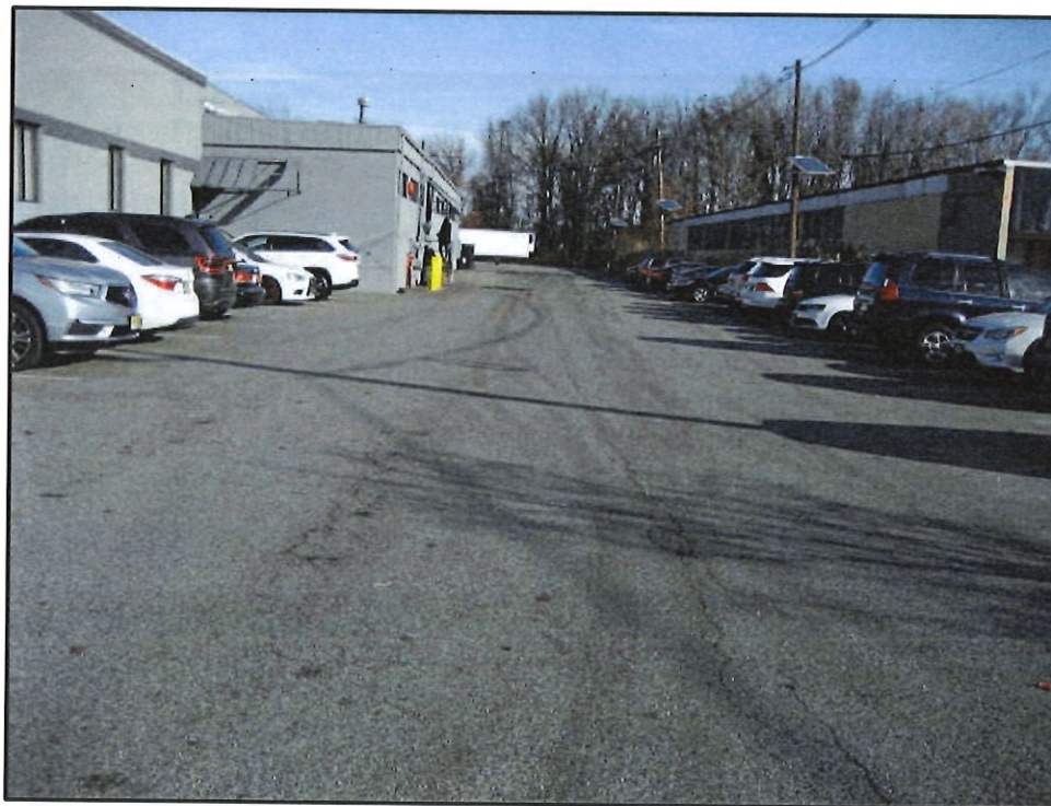
Photo 4 – Engineering Control C-2: Asphalt Cap Protective of Human Health and the Environment
