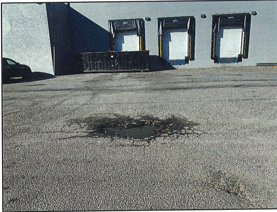
Photo 1 – Engineering Control C-2: Asphalt Cap Protective of Human Health and the Environment, but in need of repair
