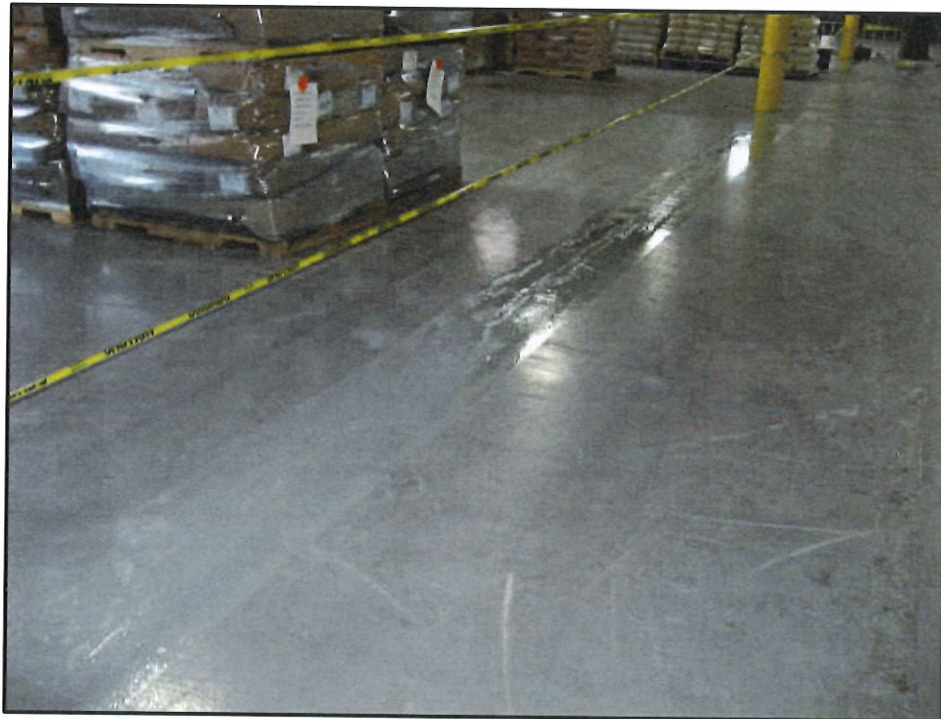
Photo 8 – Engineering Control C-3: Patched Concrete Slab (Building Foundation) Protective of Human Health and the Environment
