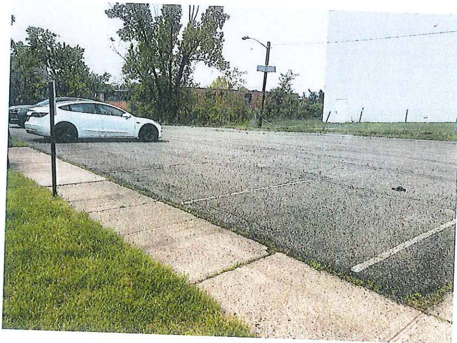
Photograph #6 – View of the asphalt cap and concrete sidewalk cap of the subject property.
